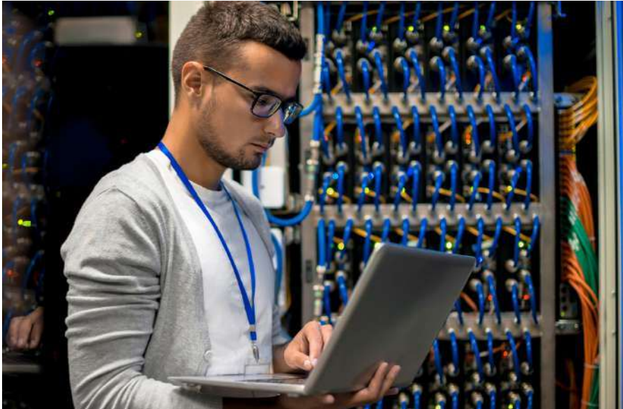
Network technician at a hospital site
